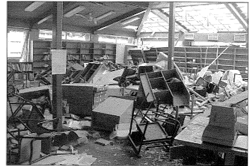
Figure 2 Anything that survived the blast inside the library was too dirty, wet, mouldy or embedded with glass to salvage
