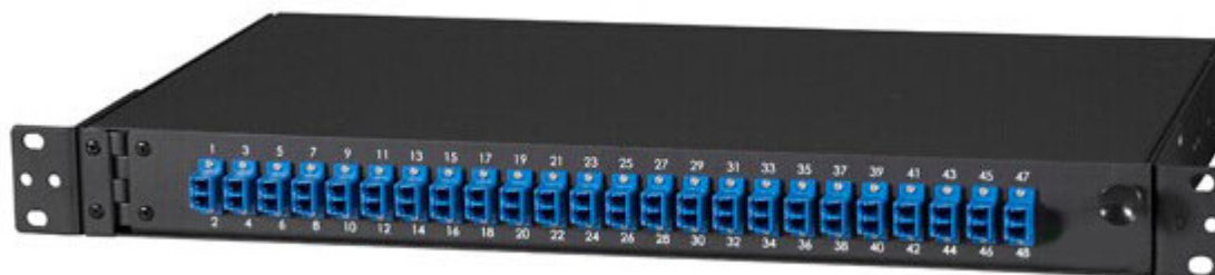
Figure 9 - Example of a high-density fibre enclosure
