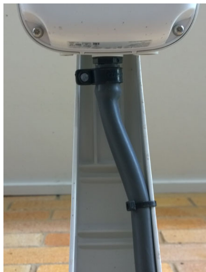
Figure 13 - External WAP installation ref. 2 (Note use of BSP fitting for cable ingress to WAP)
