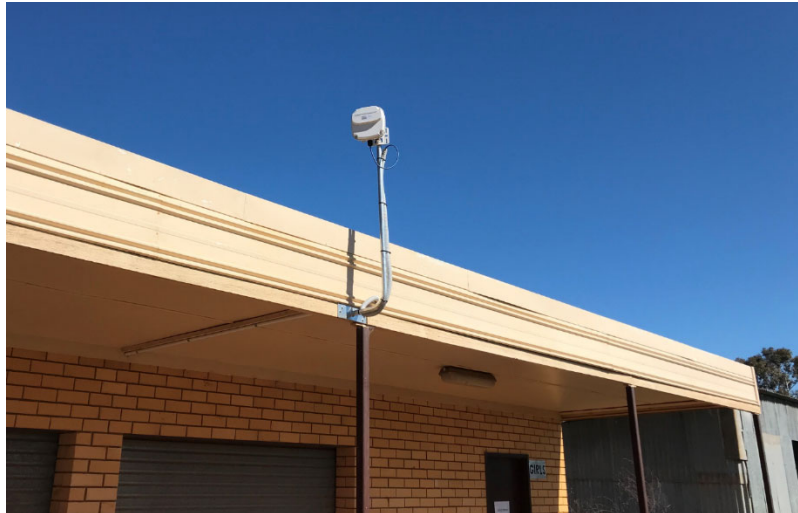
Figure 14 - Wireless bridge installation ref. 3 - BSP fitting and water proofing need to be followed as per instructions
